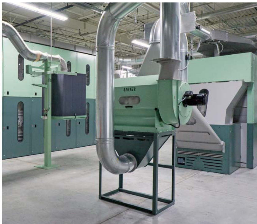
A 21 efficient tuft transport with integrated dedusting
